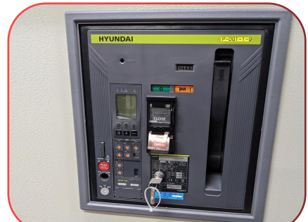
MSB Circuit Breaker
