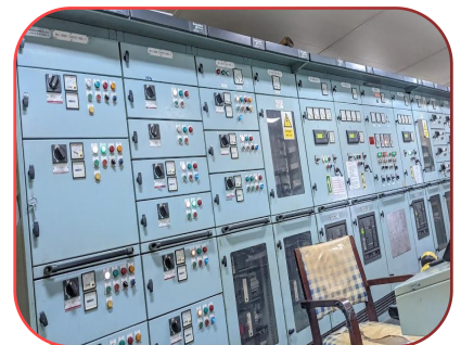
Main Switch Boards
