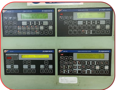
Engine Alarm Monitoring System
