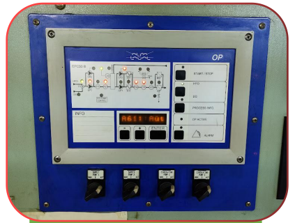
Oil Purifier Separator
