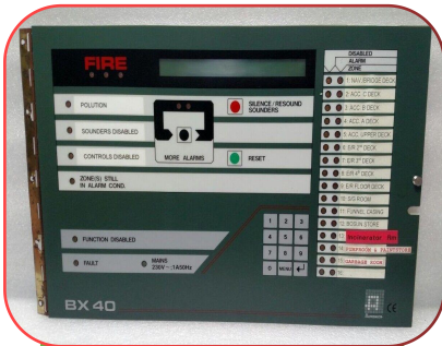
Fire Alarm Panel
