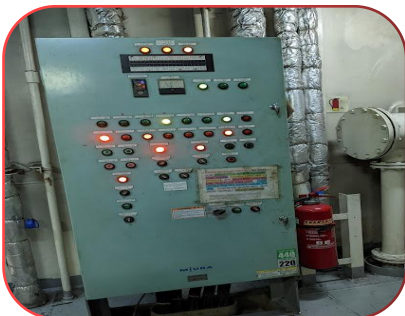
Boiler Control Panel
